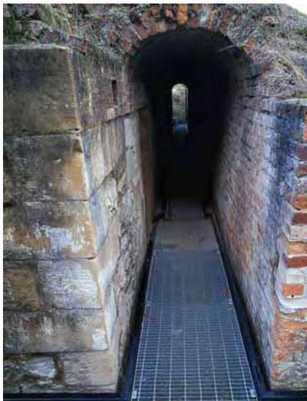
The well preserved underground cells at the Coal Mines show a high degree of integrity and authenticity.
